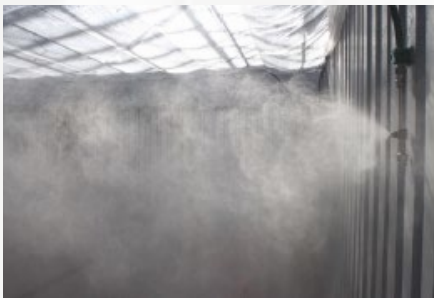
The disinfectant is sprayed from the fogging nozzles
